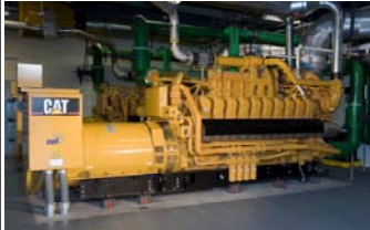
Caterpillar engine generator
