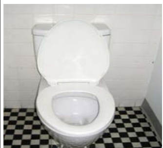
Dual Flush at Hudson's office
